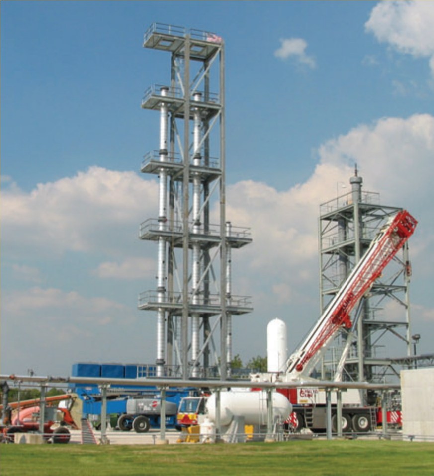
A series of propylene fractionator columns during final assembly at Diversified CPC, Channahon, IL.
